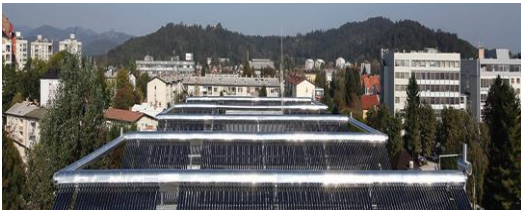
InfraSUN Ljubljana (SLO) Technology: Vacuum tube roll-bond heat-pipe collectors, silica gel adsorption chiller
