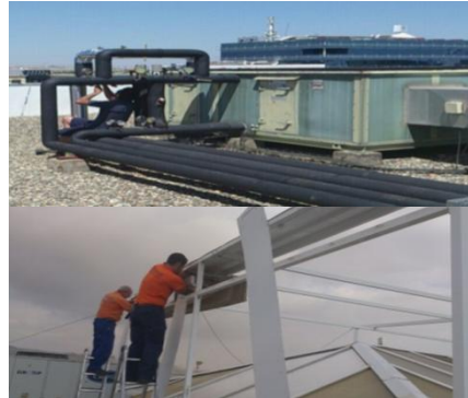
HVAC Lab Sevilla (ES) Technology: HVAC technology Lab for office buildings
