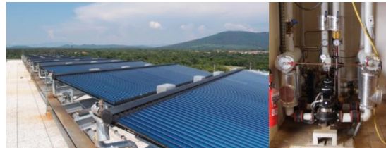
SunLab Trieste (IT) Technology: solar thermal collectors, adsorption chiller, thermal dissipater
