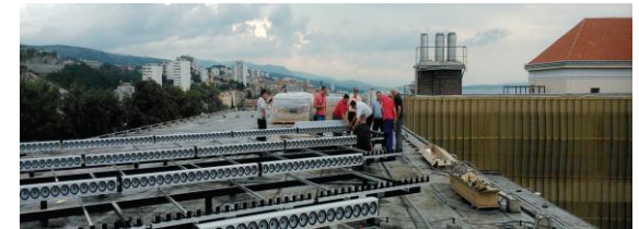
SunCool Rijeka (HR) Technology: vacuum solar collectors, ammonia-water absorption chiller
